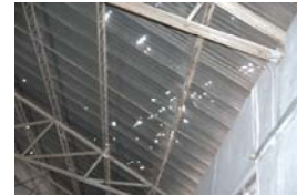
Bullet holes in roof
